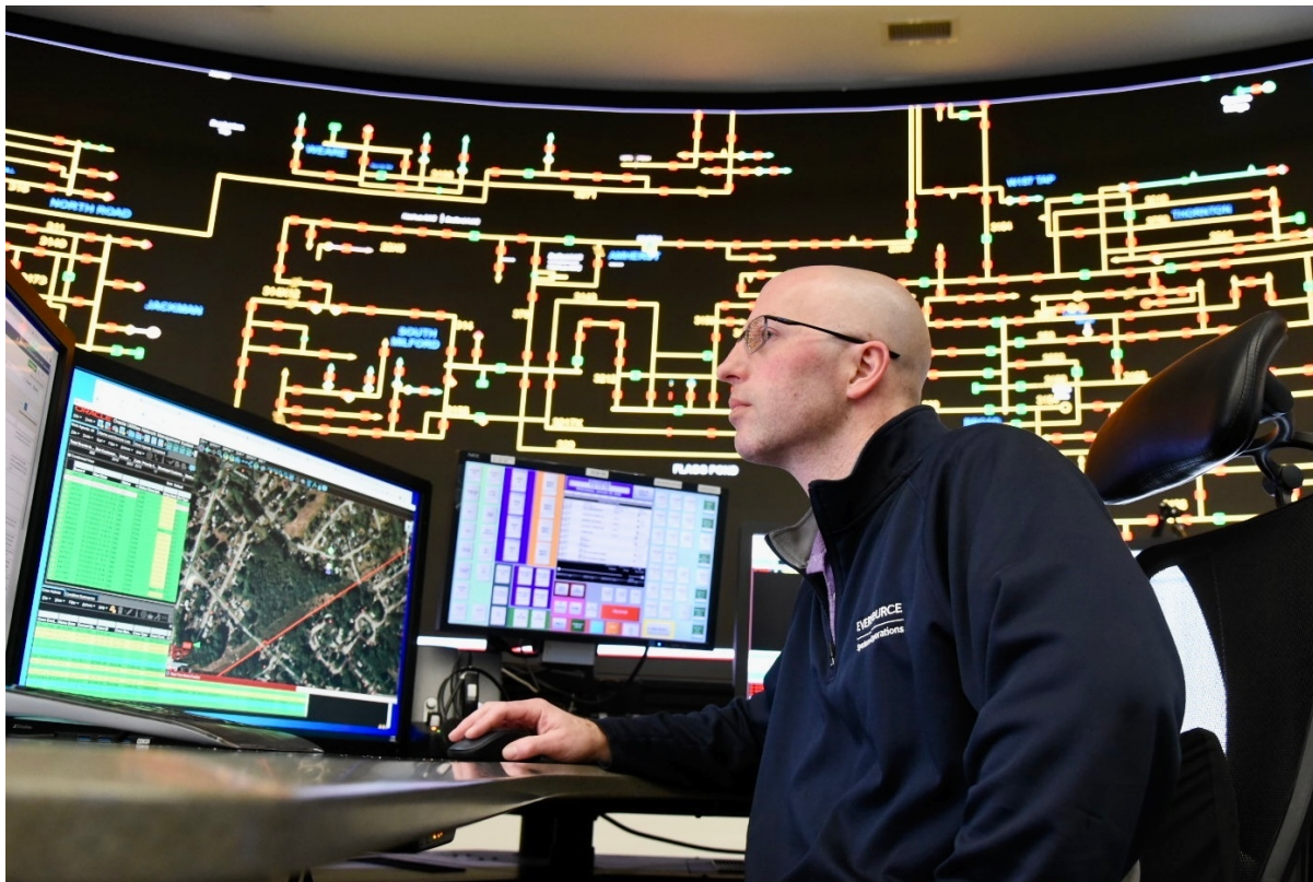
Inside Eversource's System Operations Center
